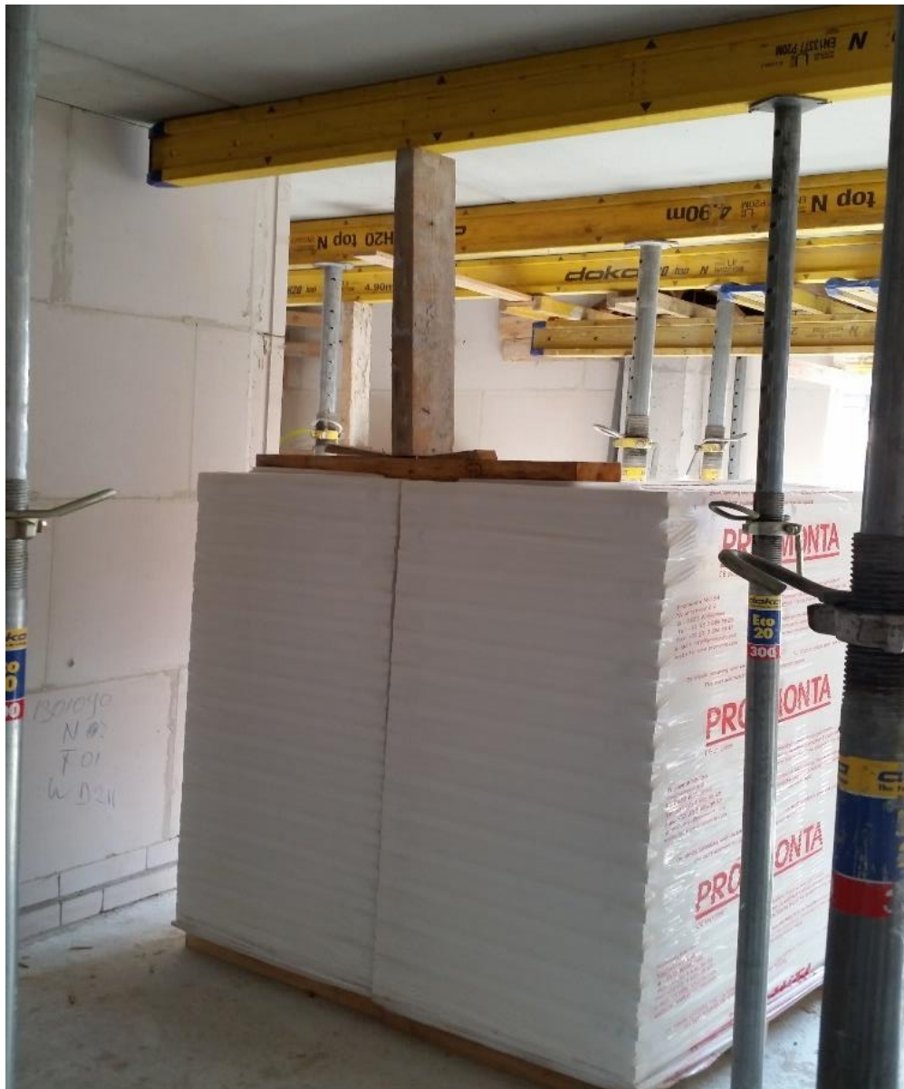
Figure 6.1.2-4 Safety issue noticed in Block 1 at beginning of the research. Risk of collapse, 3 rd floor
