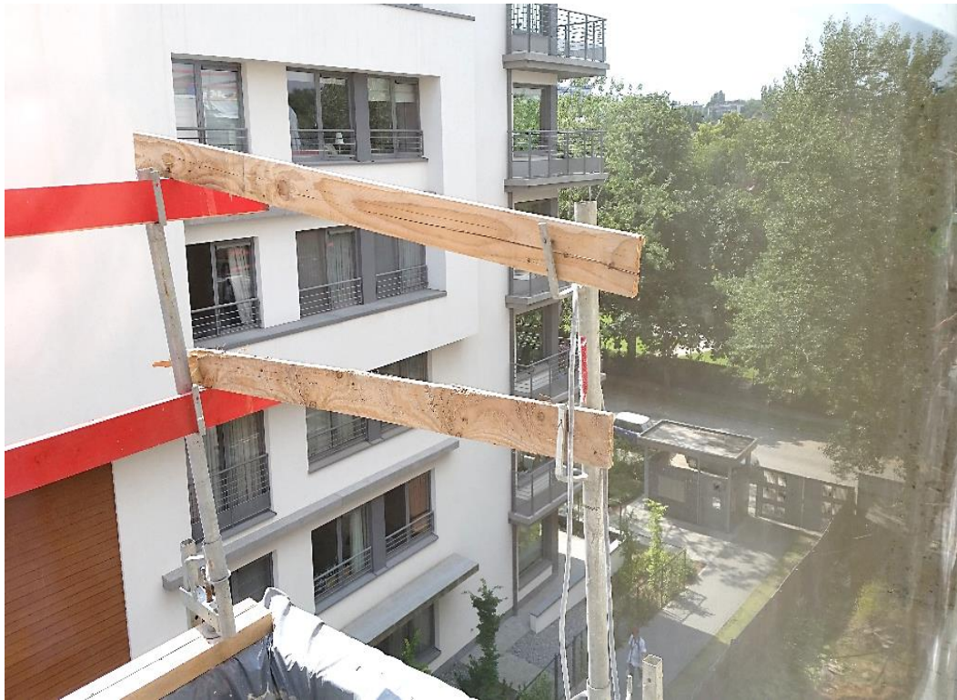
Picture 6.1.2-4 Safety issue noticed in Block 1 at beginning of the research (handrail missing)
