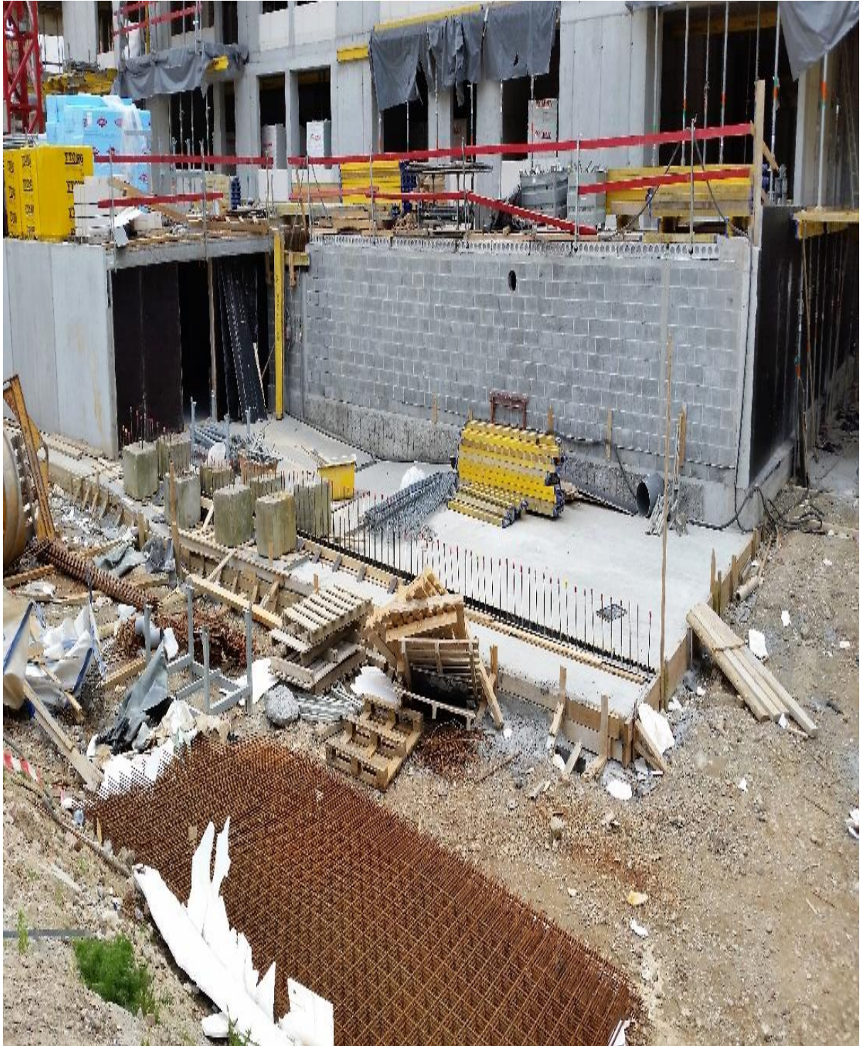
Picture 6.1.2-11 Safety issue noticed in Block 1 at beginning of the research: no pathway, iron bars unprotected, busy floor, risk of fall, ground level
