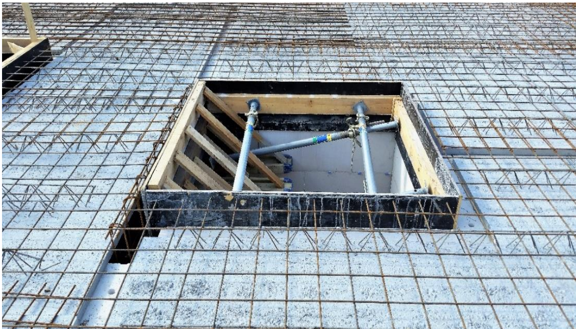
Picture 6.5.1-1 Example of safety issue (technical raisers) in block 1 (reminder)
