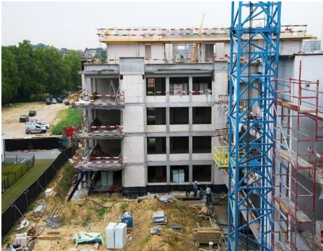
Figure 6.5.7-1-1 Illustration of the non-overlapping work sequence in the previous phases of the project (the windows were not installed before the end of the concrete works)
