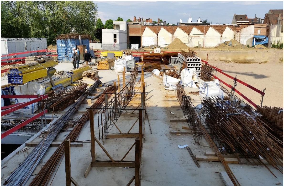
Picture 6.1.2-8 Safety issue noticed in Block 1 at beginning of the research: no pathway, iron bars unprotected, busy floor, risk of fall, ground level
