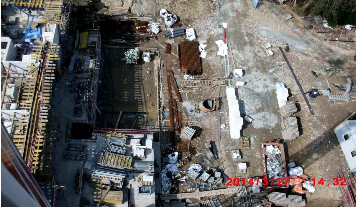
Picture 6.1.2-9 Safety issue noticed in Block 1 at beginning of the research: no pathway, iron bars unprotected, busy floor, risk of fall, ground level
