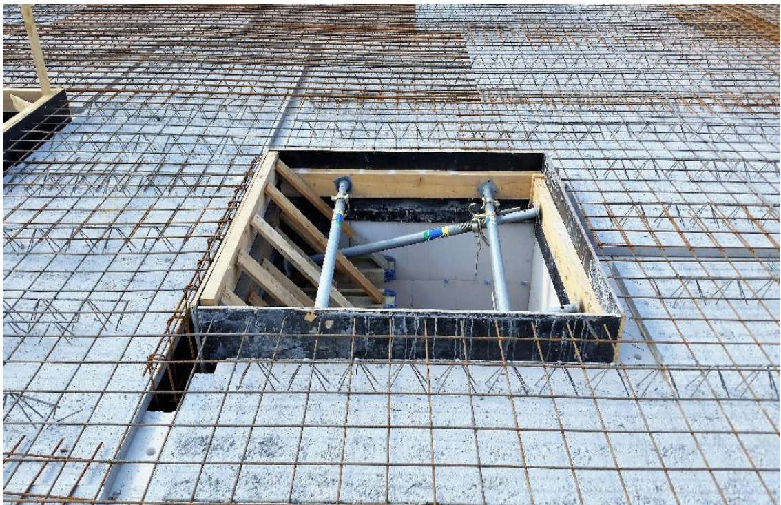
Picture 6.1.2-7 Safety issue noticed in Block 1 (anti-fall protection missing), 5th floor
