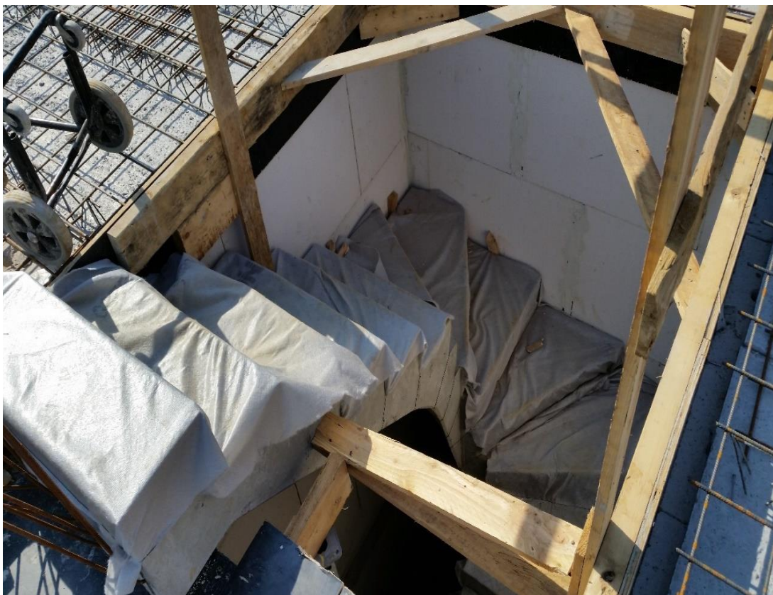
Figure 6.1.4-5 Example of safety issue in Block 1 (block1): risk of fall in the staircase, 5th floor
