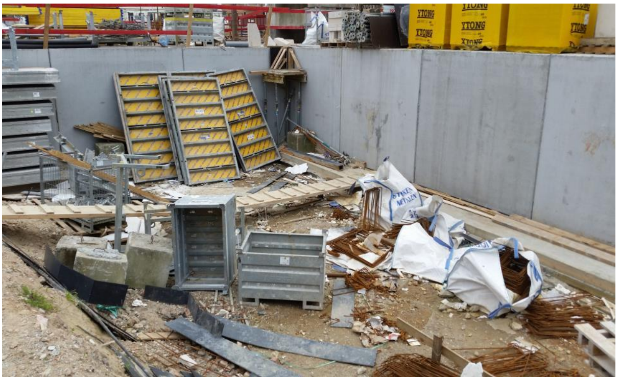
Picture 6.1.2-10 Safety issue noticed in Block 1 at beginning of the research: no pathway, iron bars unprotected, busy floor, risk of fall, ground level
